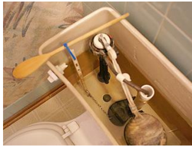
Example of supporting a "Ball Valve" float to stop overflow
