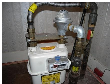
Example of a gas meter with shut of valve located on pipework (red handled lever)
